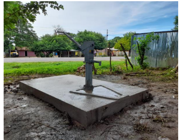
THE TEAM HAS FINISHED INSTALLING THE HAND PUMP AND POURING THE CONCRETE PLATFORM.
