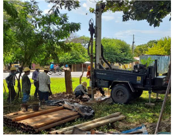
THE STAFF DRILLS A BOREHOLE DEEP INTO THE EARTH UNTIL HITTING A SAFE WATER AQUIFER.
